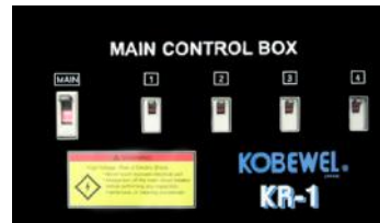
Main Control Box
